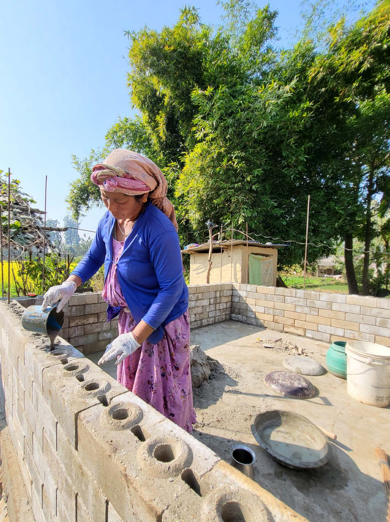
A woman builder in the process of building affordable and earthquake resistant house using Compressed Stabilized Earthen Bricks (CSEB) interlocking bricks in Kailaki district.
